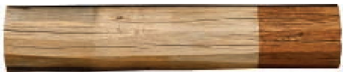
Prep method used was power washing followed by an Osborn Brush. The bare wood shown in the middle DOESN'T return to its natural color after pressure washing.
